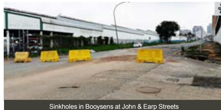
Sinkholes in Booyens at John & Earp Streets
