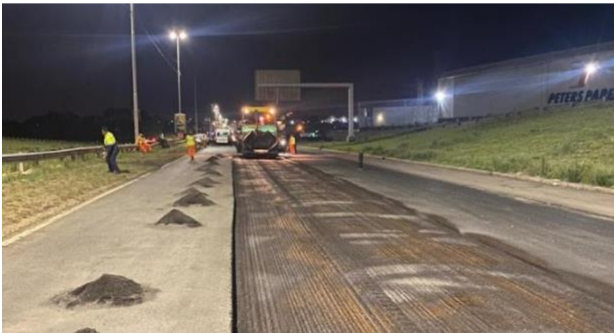
An example of some of the road works currently underway at the M2 Motorway Project
