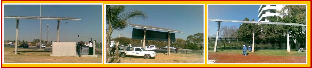
Picture: Solar Panels and battery back up for traffic signals.
